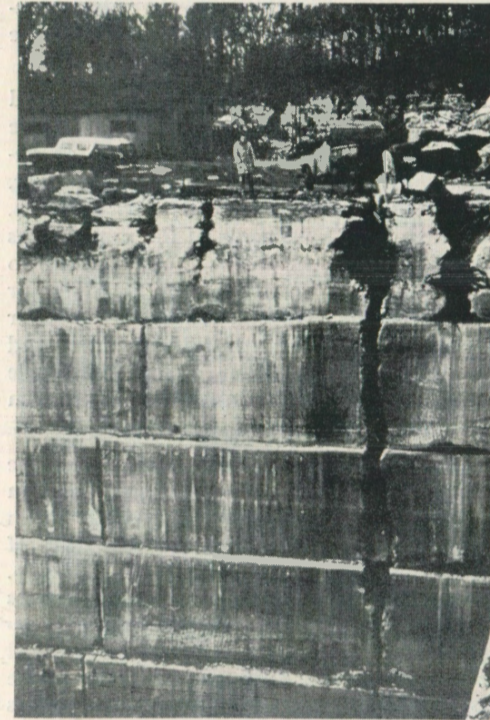
Figure 2 Joints enlarged by solution (cutters) in a quarry face in southern Indiana.
